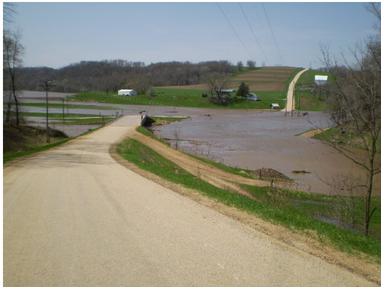
Picture 2: Camel Ridge Road Overtopping, Waterloo Township - April 25, 2008 Flood
